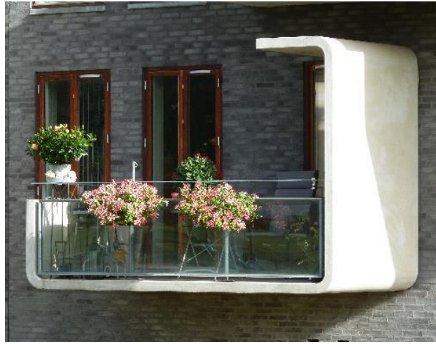
Figure 2: Cantilevered balcony element placed on corbels in the bottom of the deck and with bolted connections transferring tensile forces into the façade from the top of the balcony upstands.
